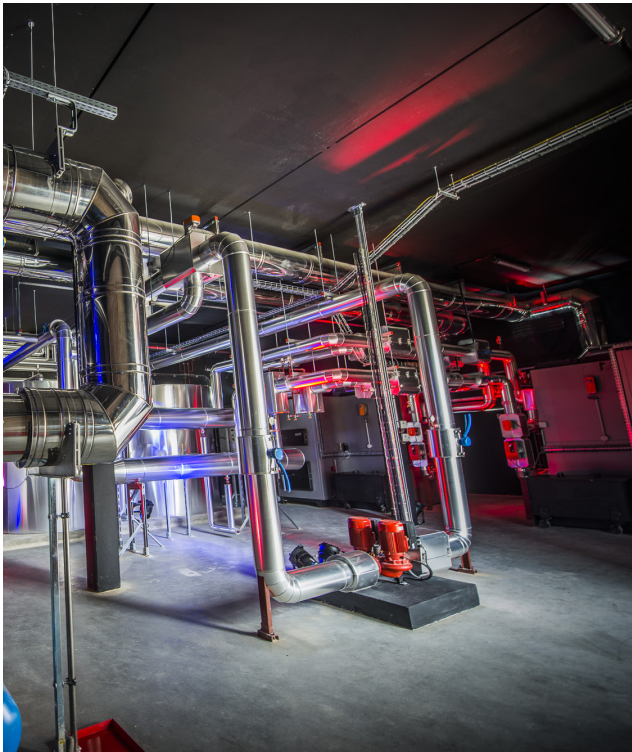
© Mission Val de Loire. The Energy Centre.
